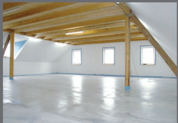
Thanks to the light weight, rapid construction progress is possible on structurally critical substrates.
